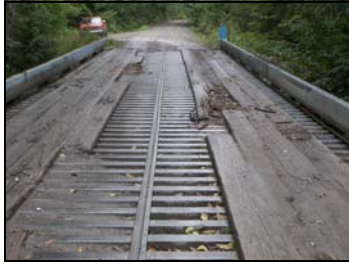
Replacing the planks on the Big Creek bridge will improve access for forest users.
